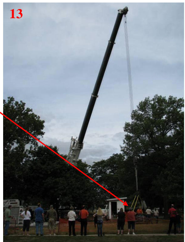
View of the crane as it tips the obelisk into the upright position.
