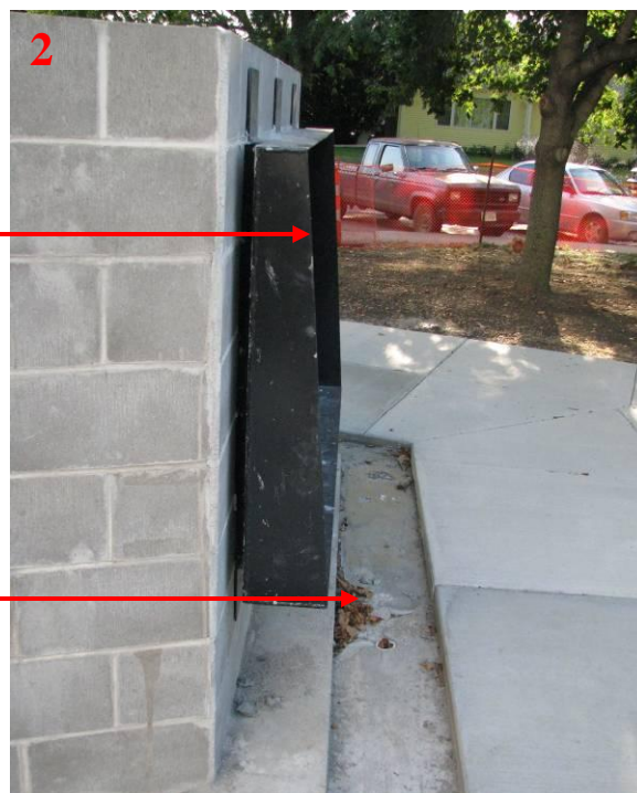
Side view of the steel box showing taper for the brick veneer profile.
