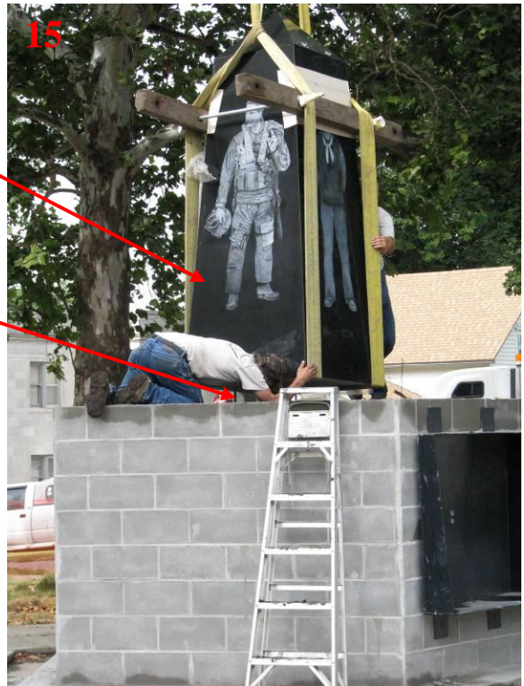
View of the workers aligning the obelisk with the foundation prior to final setting.
