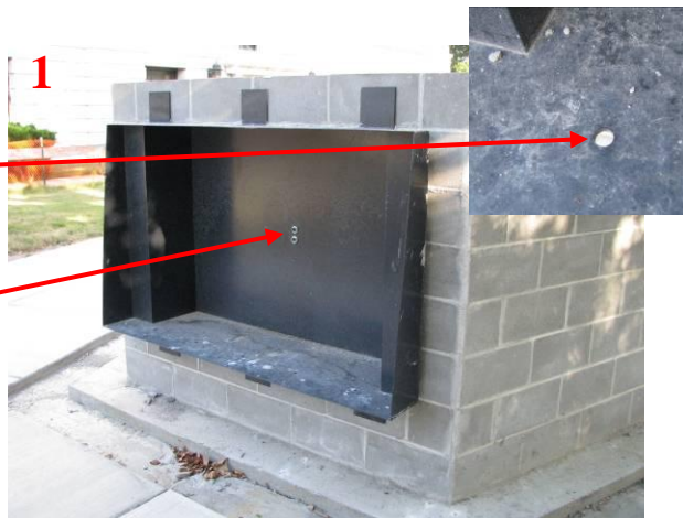
View of the steel box for the kiosk and the weep holes in the bottom face of the box.
