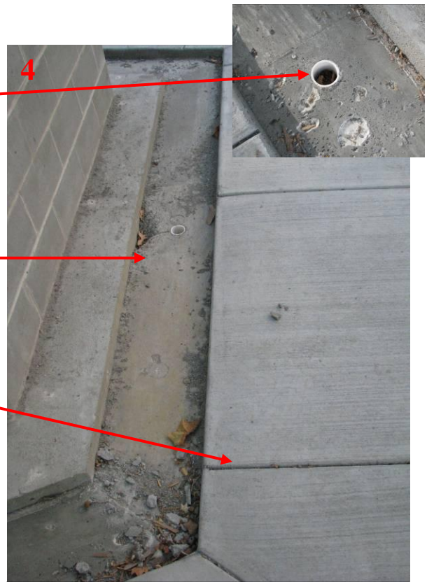
View of the slot for brick pavers and the weep holes in the base for drainage.
